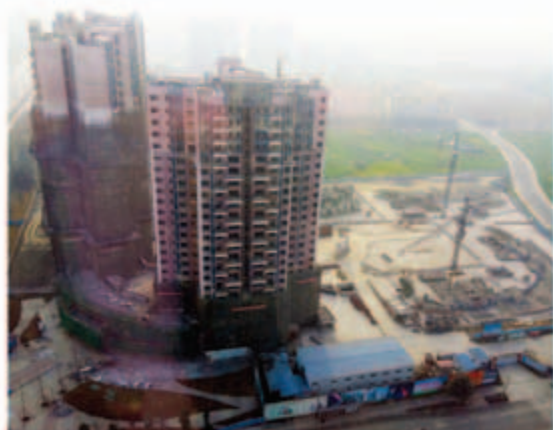
■ Three residential towers in the first stage of the composite development - superstructure works in progress
