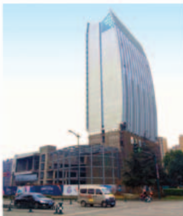
■ Regal Xindu Hotel, a five-star hotel in the first stage of the composite development - superstructure works in progress
