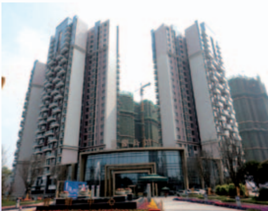
■ Three residential towers in the first stage of the composite development – nearing completion
