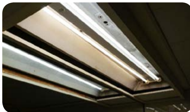
Our hotels replaced or are in the process of replacing the T8 fluorescent tubes in the guestrooms and public area with LED light tubes for further energy saving.
