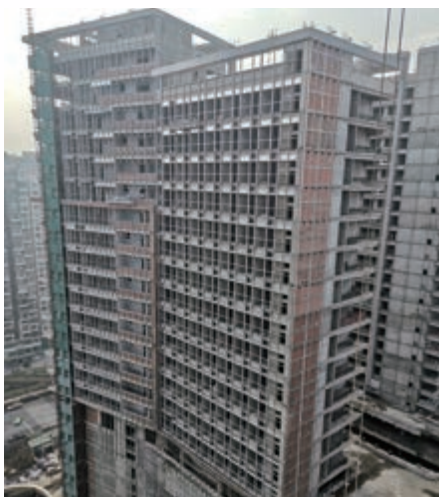
Superstructure works for the commercial/office towers of Regal Cosmopolitan City in progress
