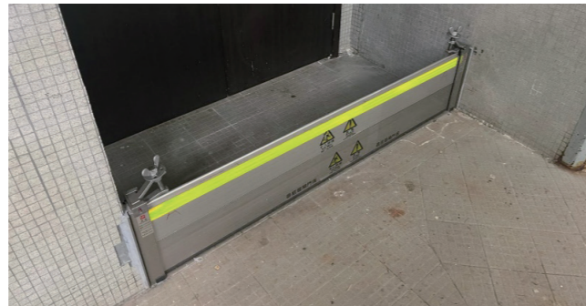
Flood Gate at Regal Airport Hotel
